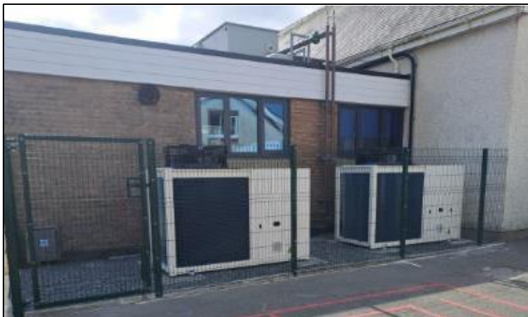
Figure 2 - Heat Pumps at Ysgol Rhosneigr
