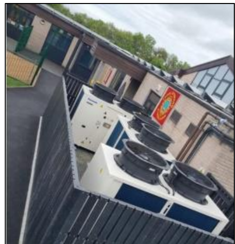
Figure 3 - Heat Pumps at Ysgol Kingsland
