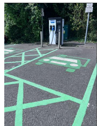
Figure 8 - New Charging Points
